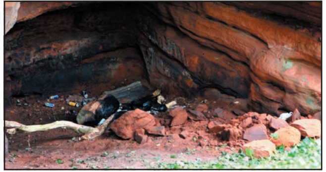
Aftermath of the roof fall in the Hermitage cave (photo: AP).
